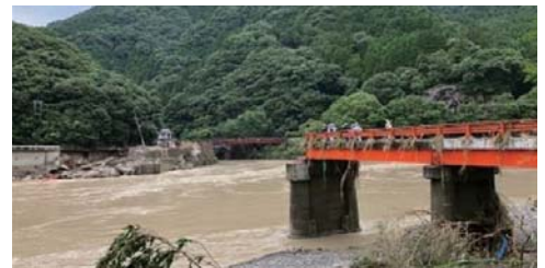
Prefederal road in Kumamoto Closed for more than four months
